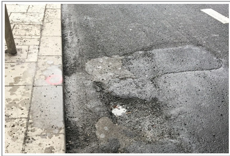
(figure4: illustration of pothole road in Thailand)
